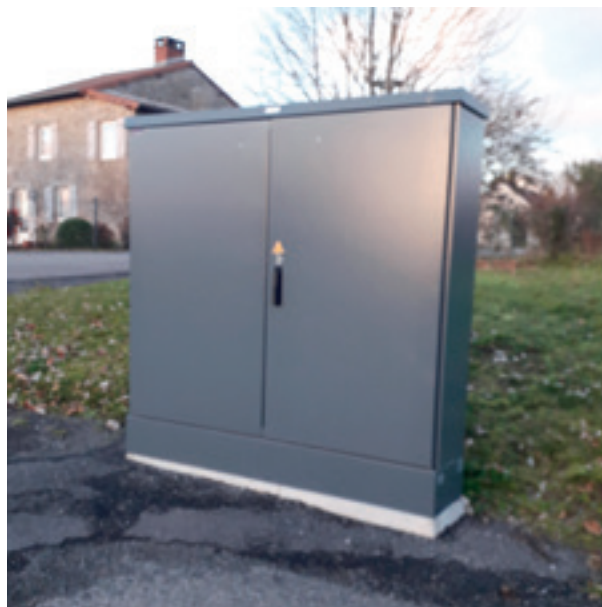
Armoire de raccordement
